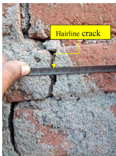
Figure 9. Hairline crack on wall
