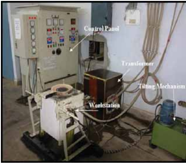
Figure 1. Induction melting furnace.
