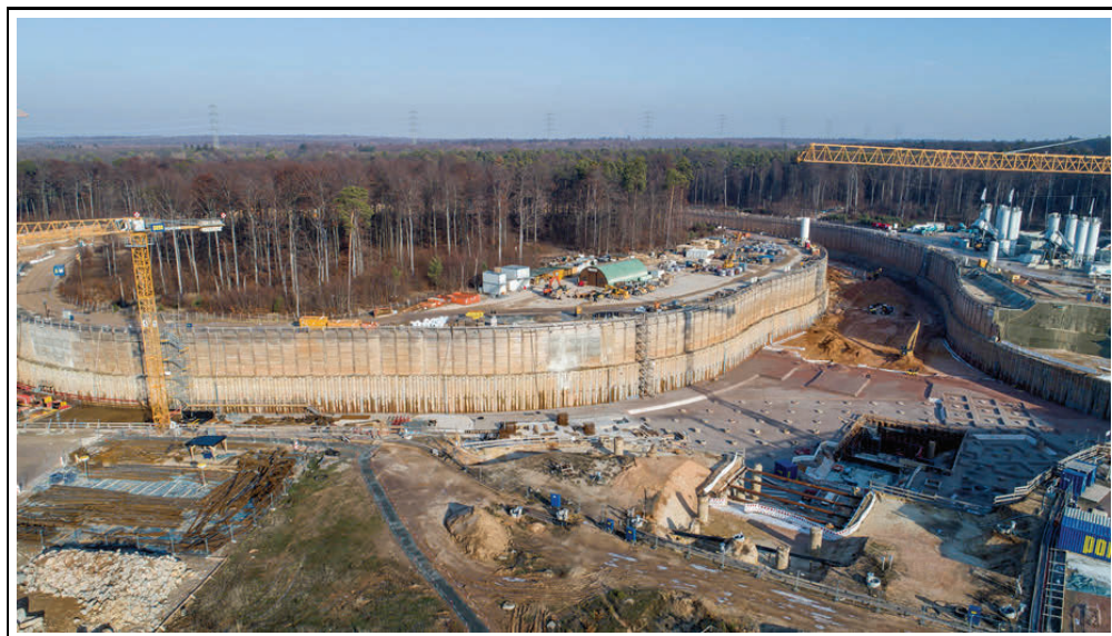
Figure 3. Aerial view of the FAIR construction site showing the excavations for the SIS100 tunnel.
