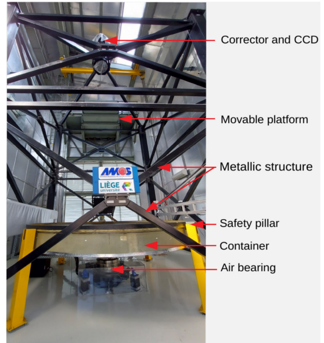
Figure 2. Inside view of the fully installed ILMT. Major components are indicated. The enclosure floor is painted with high-quality epoxy paint to avoid any spread outside the dome in case of accidental mercury spillage.
