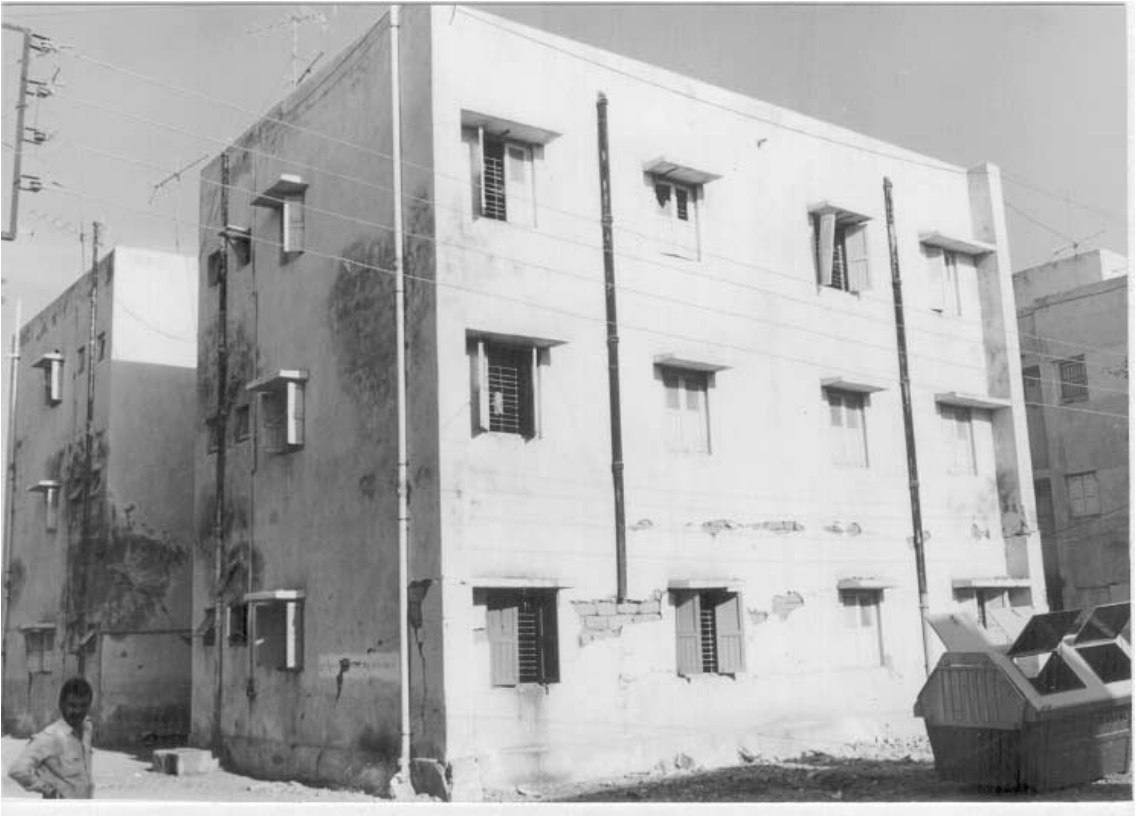
Figure 4. Stone masonry building in CM with minor damage (Bhuj).
