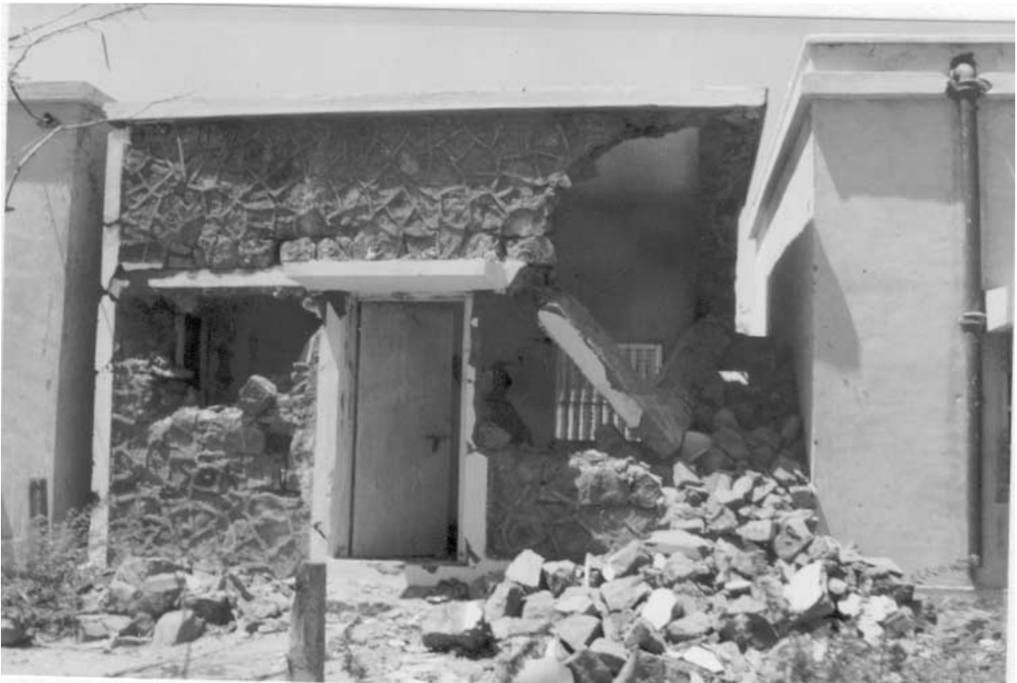
Figure 5. Out-of-plane failure of wall leading to collapse of lintel band (Bhuj).
