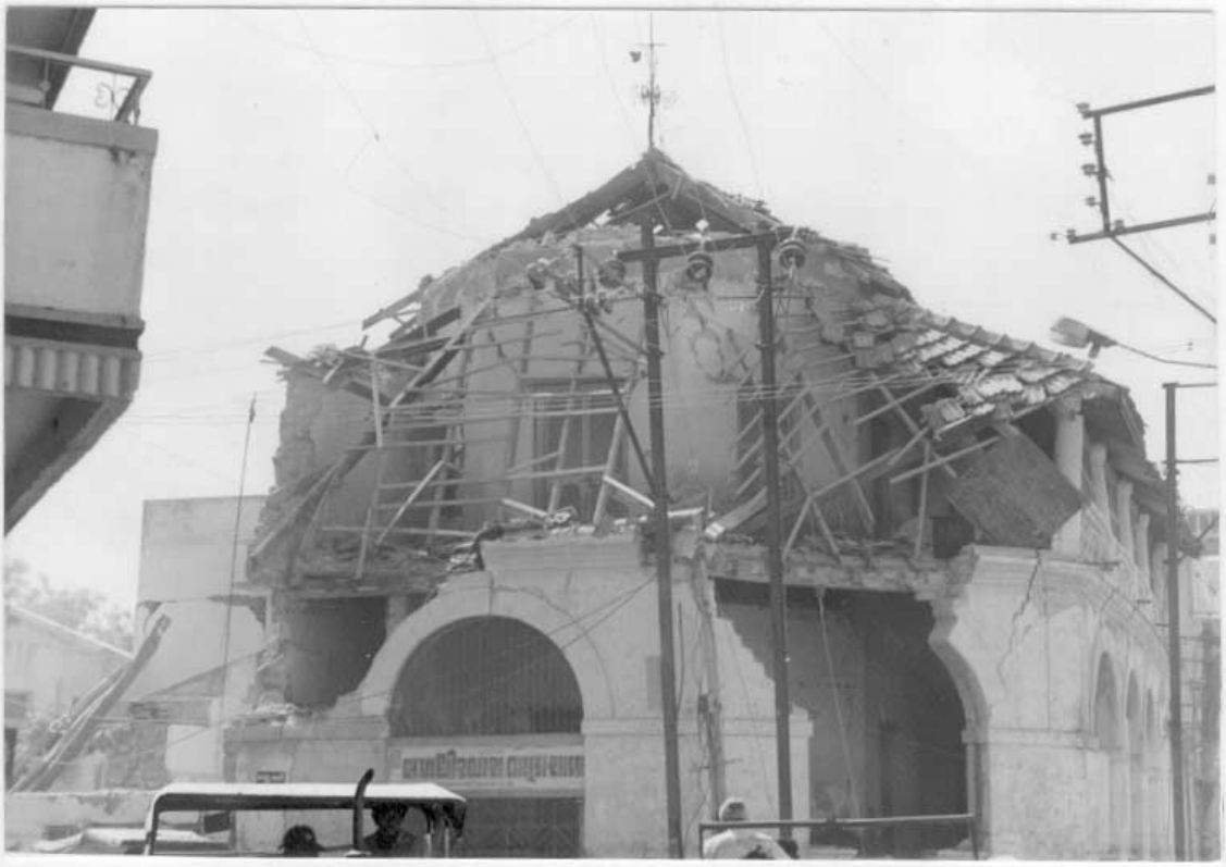
Figure 1. Out-of-plane collapse (Morbi).
