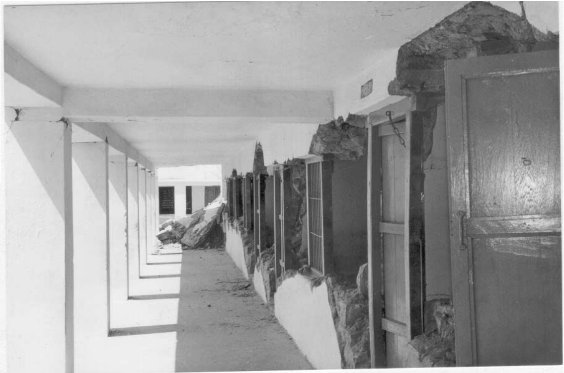
Figure 7. Collapse of wall between openings (Khavda).
