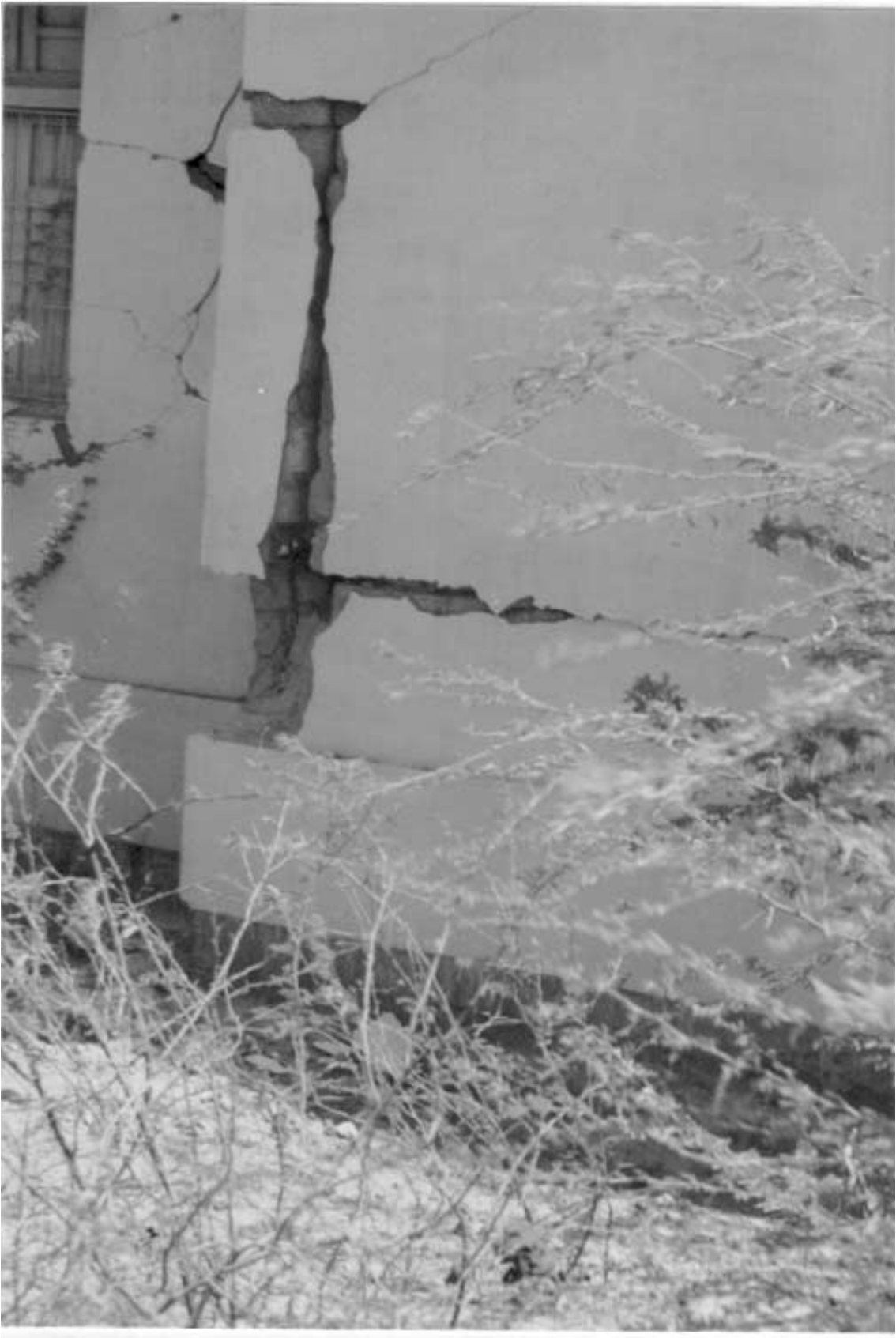
Figure 6. Corner failure in the presence of corner reinforcement (Bhuj).
