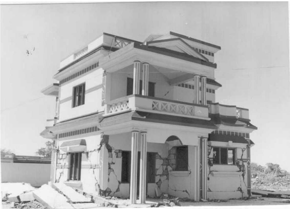
Figure 2. House with lintel band and corner columns, cracks below band (Samakhyali).
