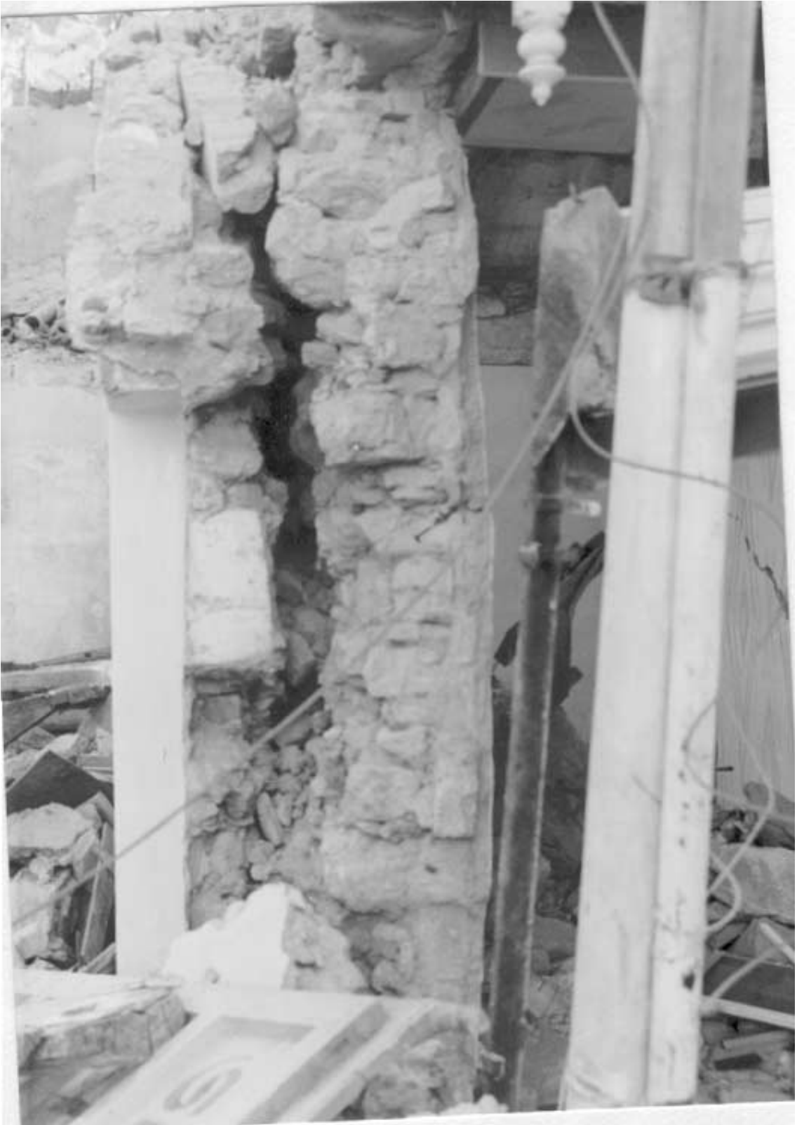
Figure 10. Delaminated wall with buckled wythes (Anjar).
