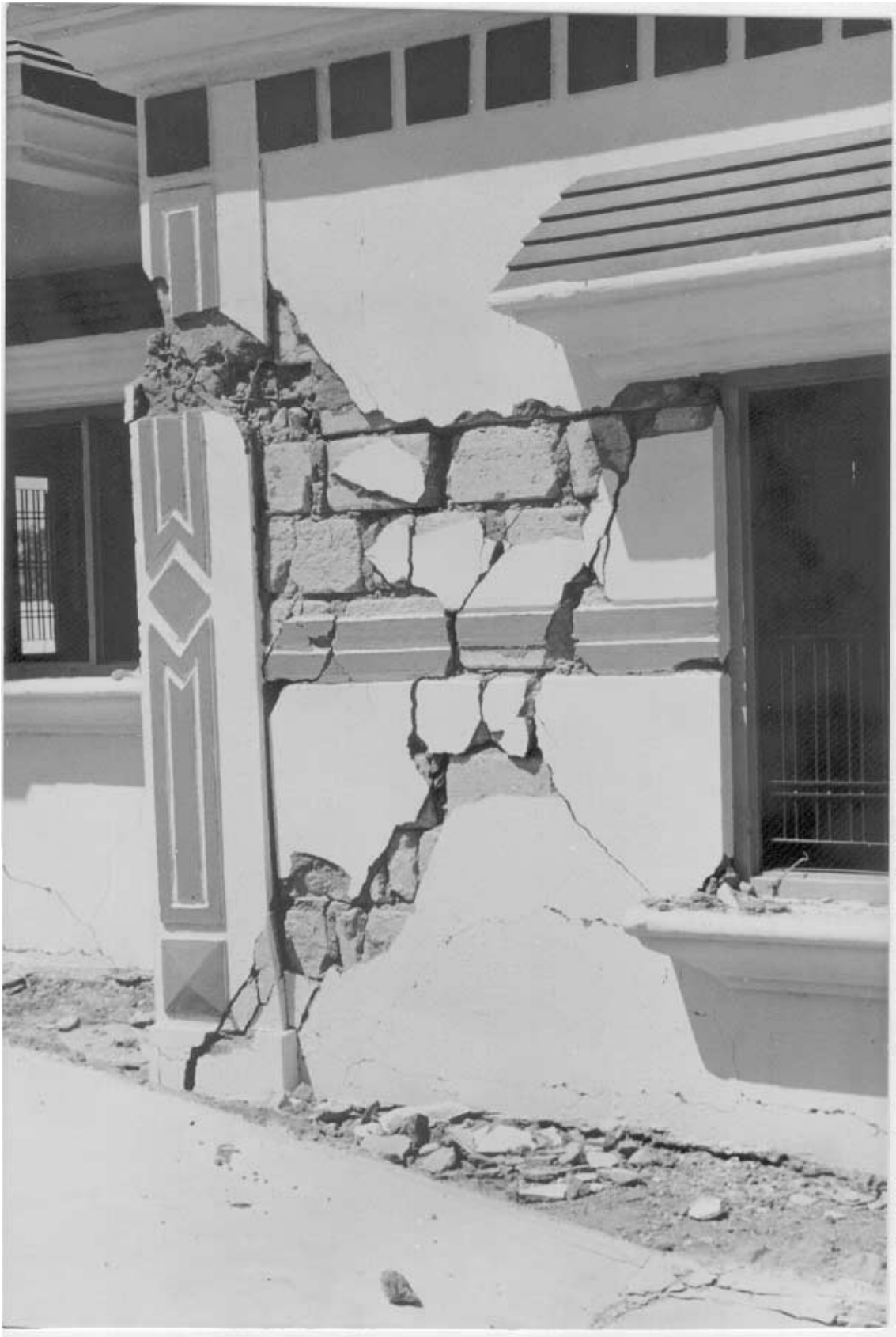
Figure 3. Wall separated from column (Samakhyali).
