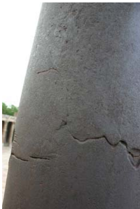
Figure 9. Side view of the pillar at the cannon ball strike location showing deflection of the horizontal crack from the rear (right side of the image) to the axial direction of the pillar by cracking of lump–lump interface.
