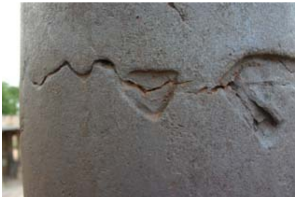
Figure 8. Close-up view of the triangular-shaped spalled region on the rear side.
